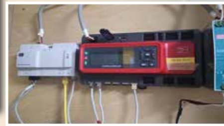
The brain of the system that sends information to a computer for monitoring
