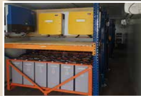
72 storage batteries for 82.56 kW solar PV system, the blue box supplies the university and the two yellow boxes supply the Faculty of Science and Engineering offices when there is EEC power cut
