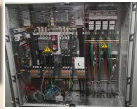
The multi cluster control box for the solar PV system
